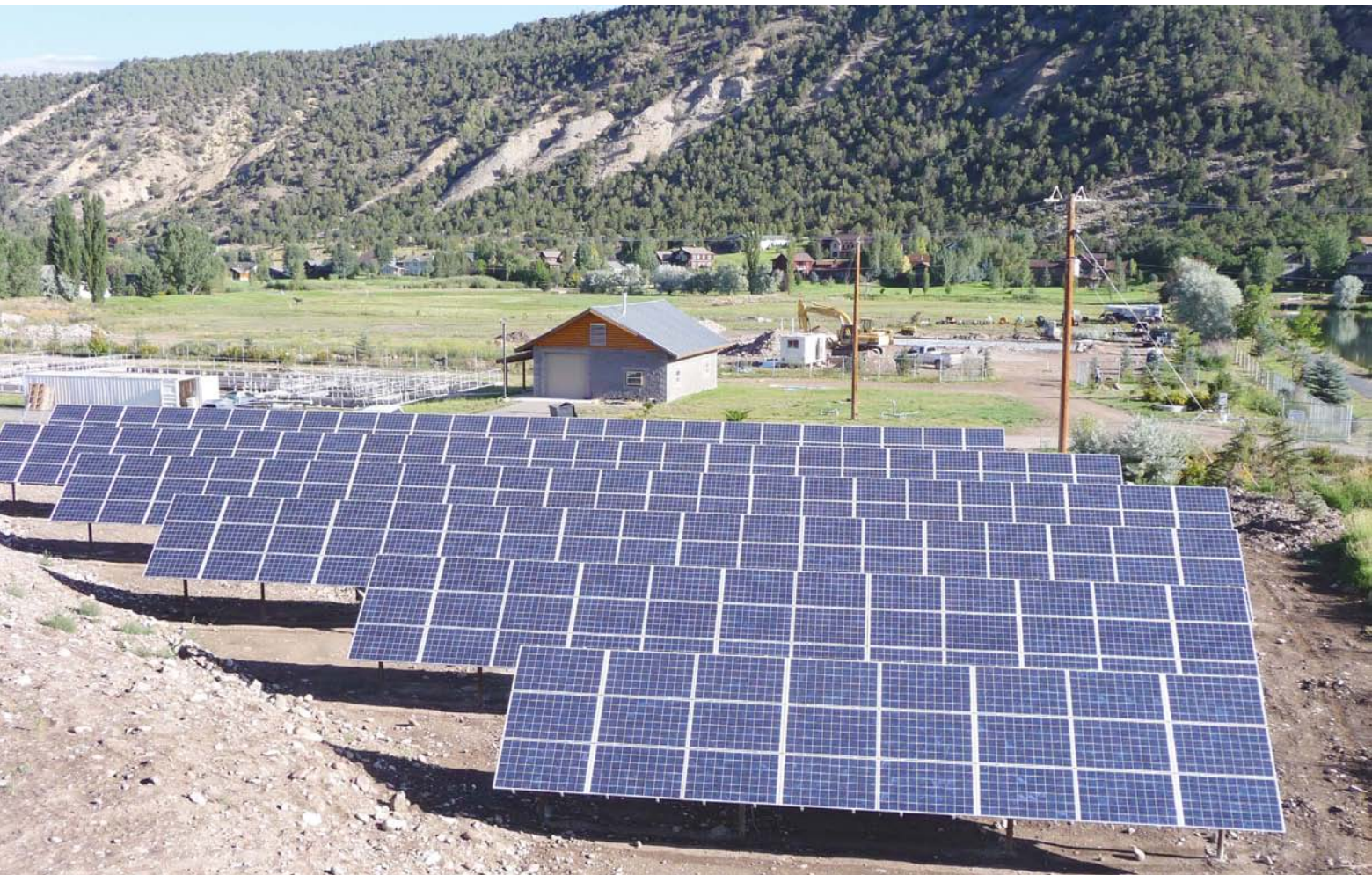
The CEC's first member-owned PV array in El Jebel, Colorado.
